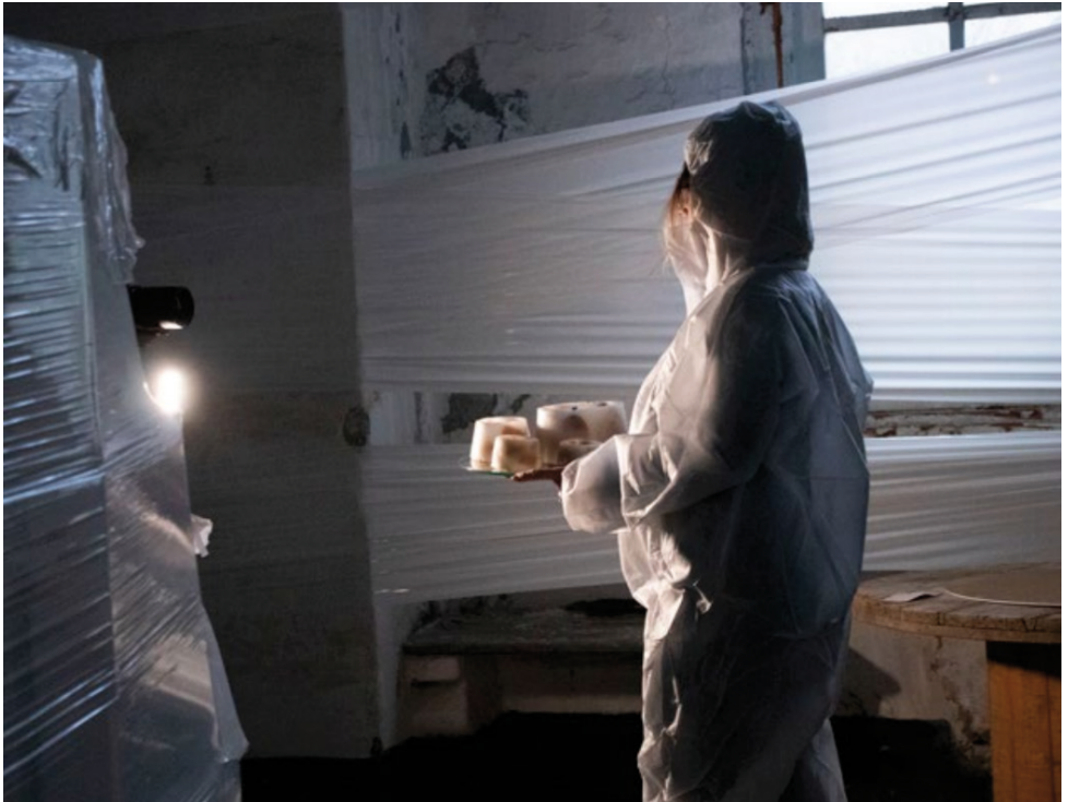
Interior space: Women's Corridor, a wing of the Albergo still under renovation. ▲
